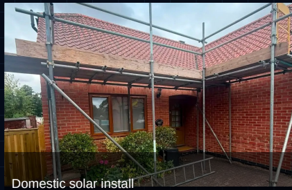
Domestic solar install
