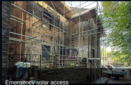
Emergency solar access
